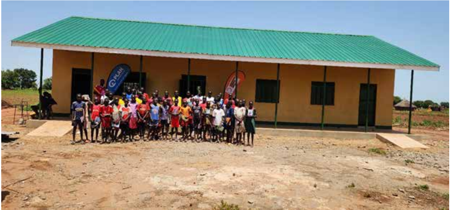
A picture of the classroom construction, on the finishing stages, about to be handed over to the school community.
